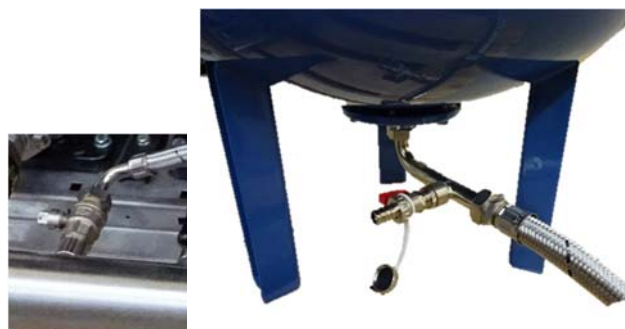
Fig. 1.3a & b Isolation valve on system pipework & Flexible hose with drain cock on vessel (non-flow through vessel shown)
